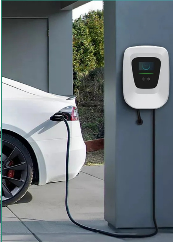
EV CHARGING WALLBOX & PILE
